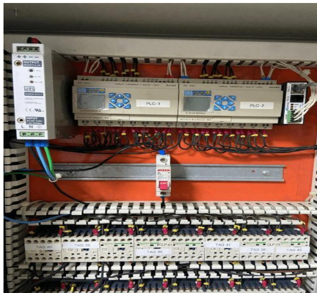
Figura 6: Painel dos CLP's e Bridge
